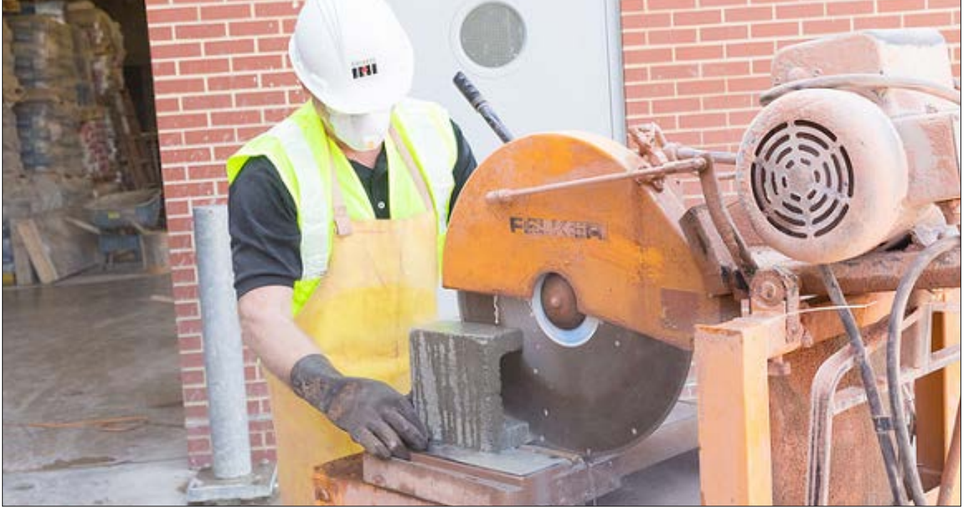
A worker uses proper protection to avoid breathing harmful silica dust while cutting concrete.
