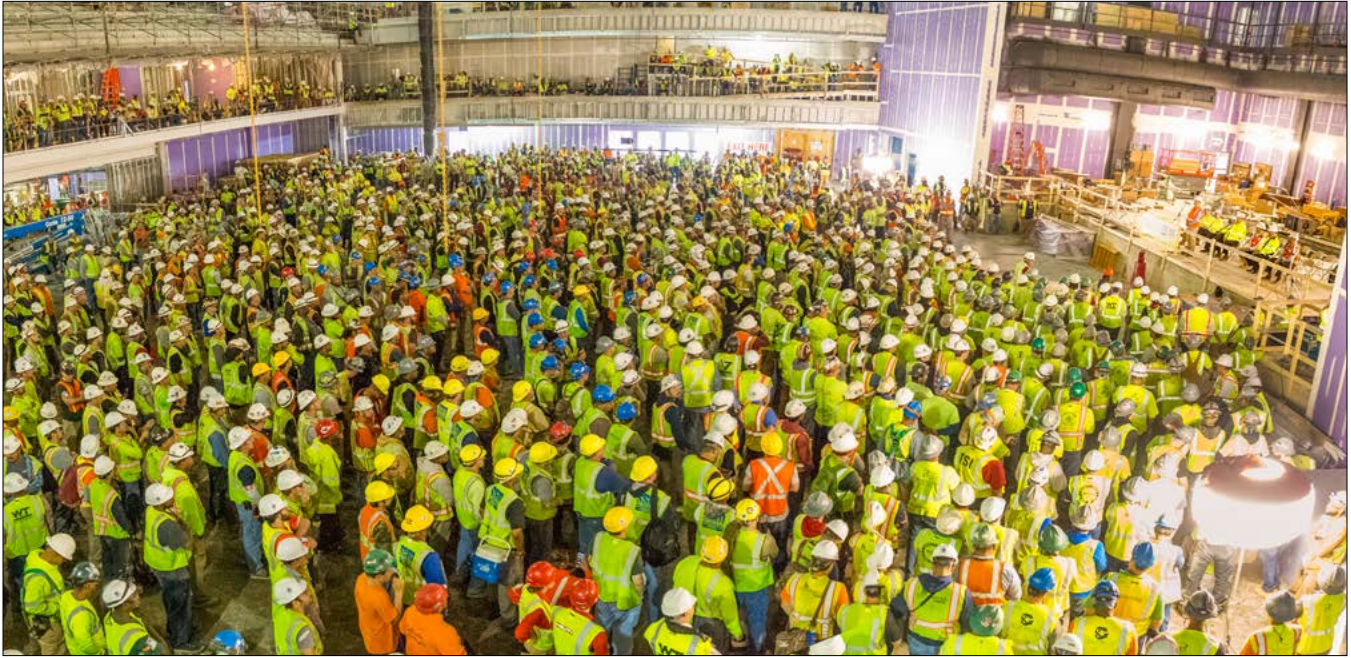
Workers at the MGM casino construction project at National Harbor stand down for safety on May 3, 2016
