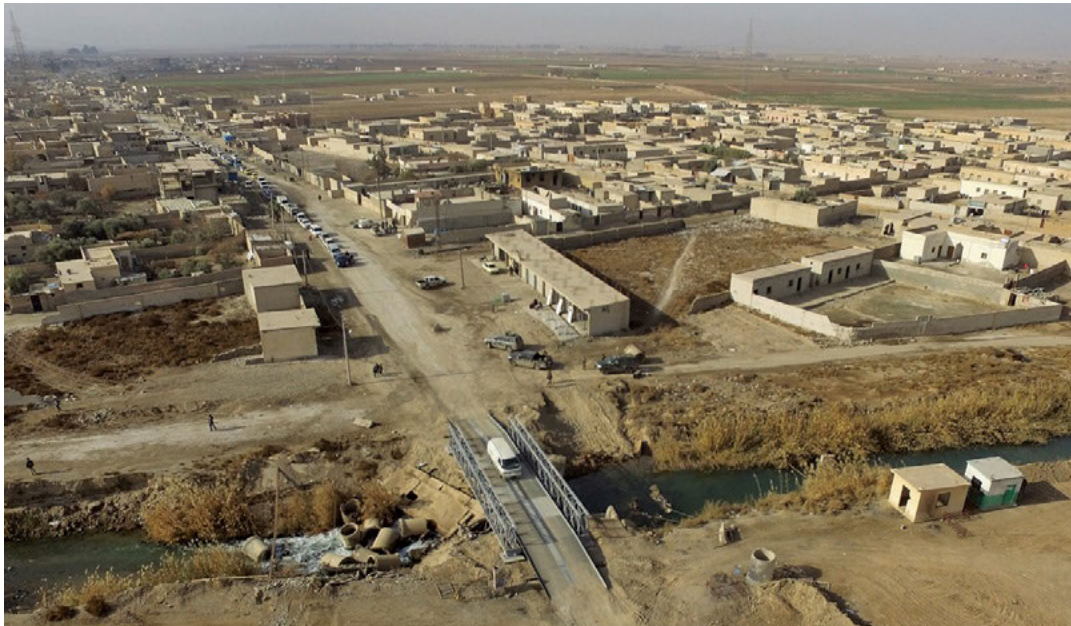
Engineers attached to the Special Operations Joint Task Force-OIR erected a bridge over the Euphrates River in the Raqqah district, Syria. (Special Operations Joint Task Force-OIR photo)
