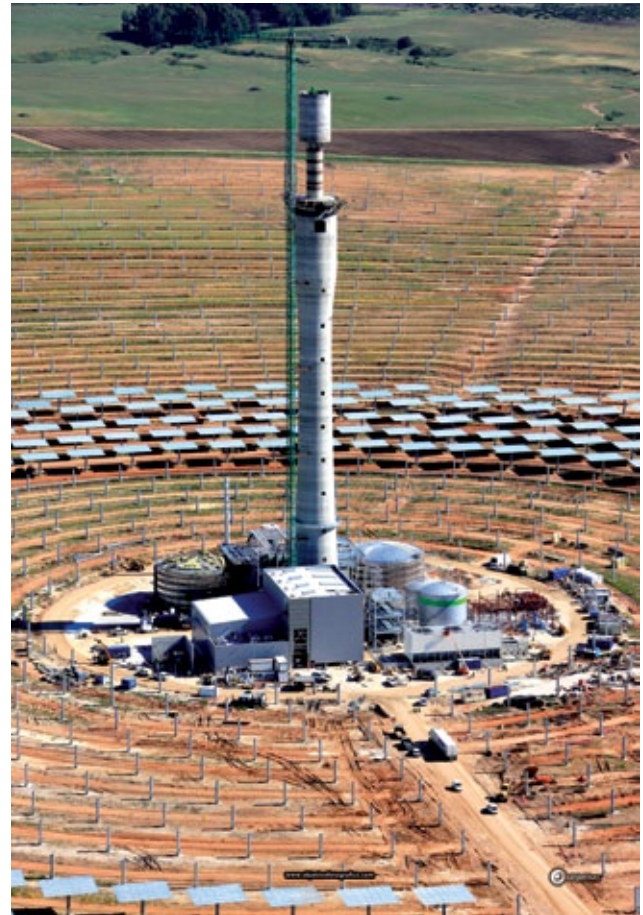
Torresol Gemasolar solar thermal power tower under construction, May 2010 SOURCE: TORRESOL ENERGY
