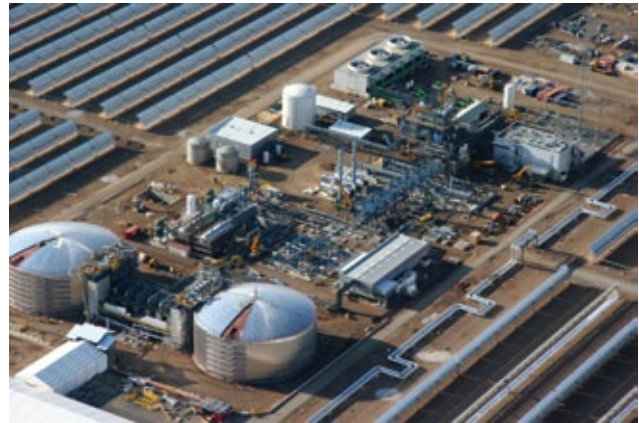
Molten salt storage tanks, Andasol 1, Spain
